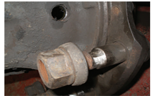
Wear To Studs
