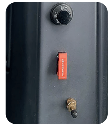
Emergency cut off switch
